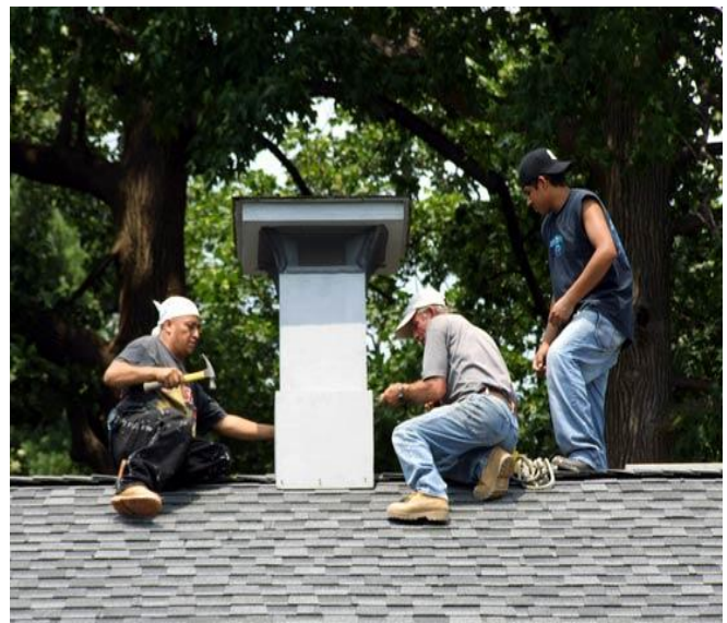
Workers from George Haag Construction Co. install a chimney vent on the roof peak of Maywood Station on July 3, 2006. The chimney vent was fabricated to replicate one that was originally found on Maywood Station in the 1872 to 1920's period. (Photo by Ed Kaminski)
