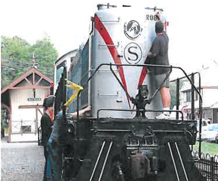
MSHC members Joe and Vince Molodowec discuss some metal work that they are about to engage in on NYS&W S-2 #206 as Ed Kaminski finishes up painting the front numbers at the July 22, 2009 work session. The 67-year old locomotive required intricate metal work in several areas to restore it to as-new condition. By the middle of September, the MSHC had finished the majority of the exterior restoration on NYS&W S-2 #206 and work had begun on restoring the interior of the locomotive cab. Future work may involve lighting the cab interior, headlights and number boards. (Photo by Robert P. Pisani)
