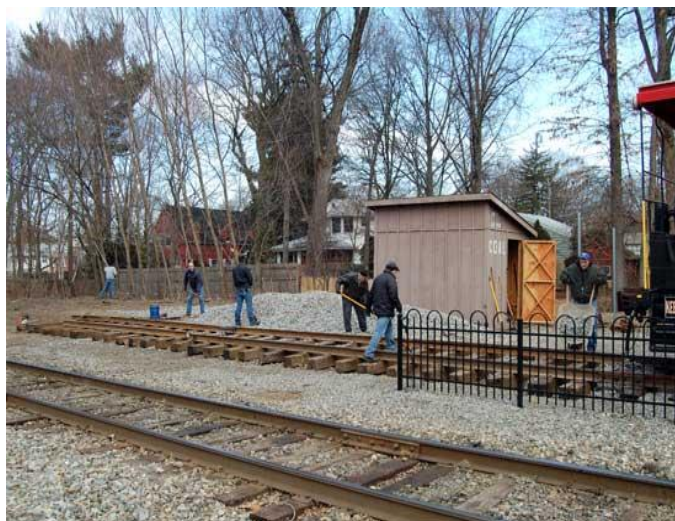
A work session was held on January 27, 2008 to install ballast for the new panel track extension and beautify the grounds including tree trimming, brush cutting and landscaping. (Photo by Keith Smollin)
