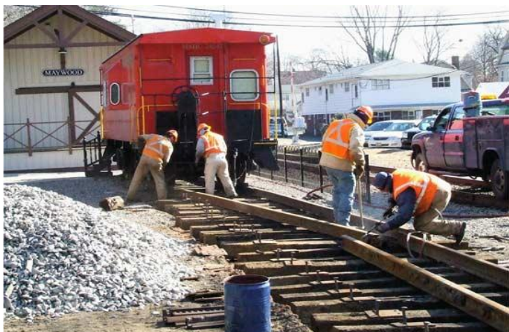
On January 25, 2008, a NYS&W track crew installed the panel track extension at Maywood Station. (Photo by Matthew Greco)
