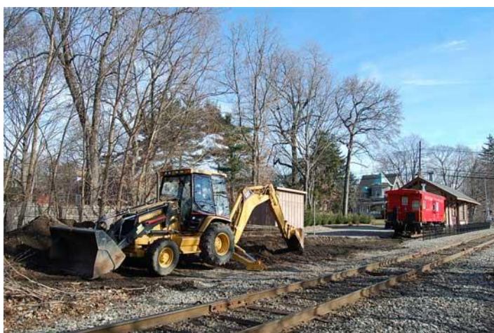
On January 13, 2008, the MSHC held a work session at Maywood Station to prepare the site for the upcoming move of NYS&W #206 into Maywood Station. Peter Scanel offered his assistance and brought his backhoe and graded the grounds as well as moved the "Coal Shed" into its new location. Looking toward Maywood Station, the grading work for the panel track extension for NYS&W #206 is nearly completed. (Photo by Tim Moses)
