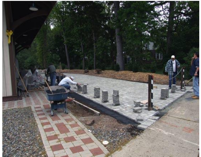
A May 11, 2006 view of A. Lepore & Grandson Masonry workers installing the new Brussels Blocks at the driveway side of Maywood Station. The station is now 100% handicap accessible inside and out. (Photo by E. S. Kaminski)
