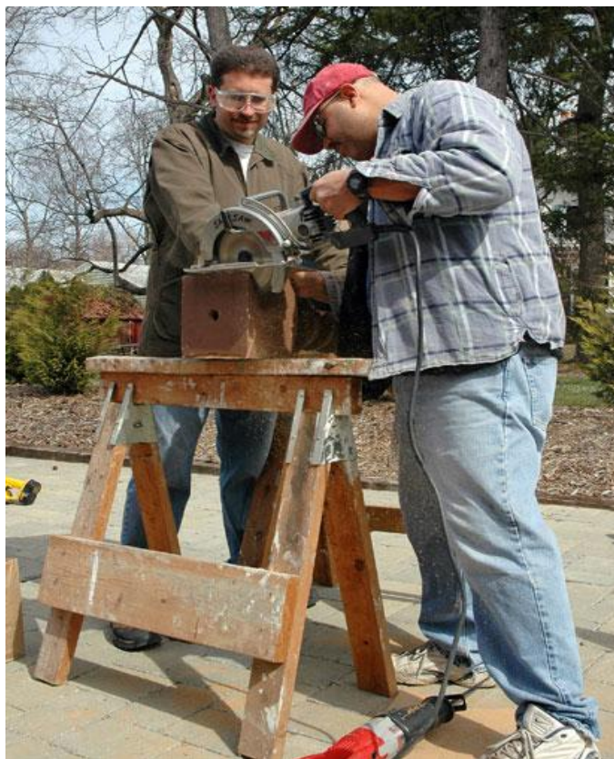
MSHC members Rob Pisani and Hector Hernandez, Jr. work on cutting a profile into the base of one of the two new finials being applied to Maywood Station's end roof peaks at the March 31, 2007 work session. The angle of the profile was very important to ensure an exact fit on the roof peak. (Photo by Doug Earls)
