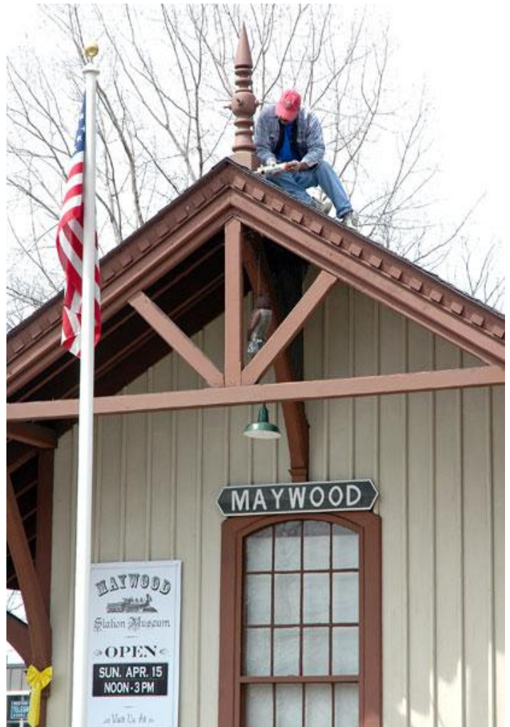
MSHC member Hector Hernandez, Jr. applies the finishing touches on the new finial at the front roof peak of Maywood Station at the March 31, 2007 work session. The intricate looking finials are a fine example of the detail MSHC members are committed to. (Photo by Robert P. Pisani)
