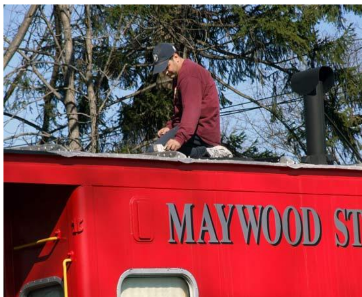
MSHC member Matthew Greco is shown applying the new silver paint system on the roof of Caboose 24542 at the March 29, 2007 work session. (Photo by Ed Kaminski)
