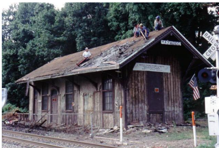
On July 24, 2002, stabilization of the roof commenced and all existing roofing shingles were removed to the bare roof. Most of the exterior stucco has also been removed. (Photo by Ed Kaminski)
