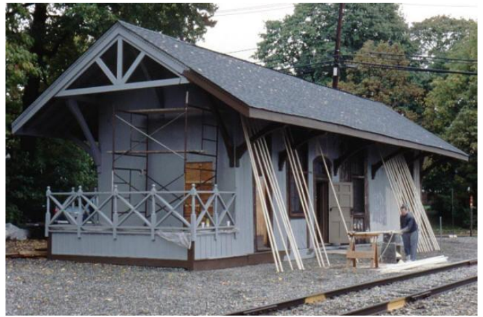
Completed battens stand in waiting for application on the south side wall while others are being cut and mitred through a saw to the original specifications by MSHC member John Tammi in this October 26, 2002 view. By winter, all battens would be applied to the station walls. (Photo by Rosemarie Kaminski)
