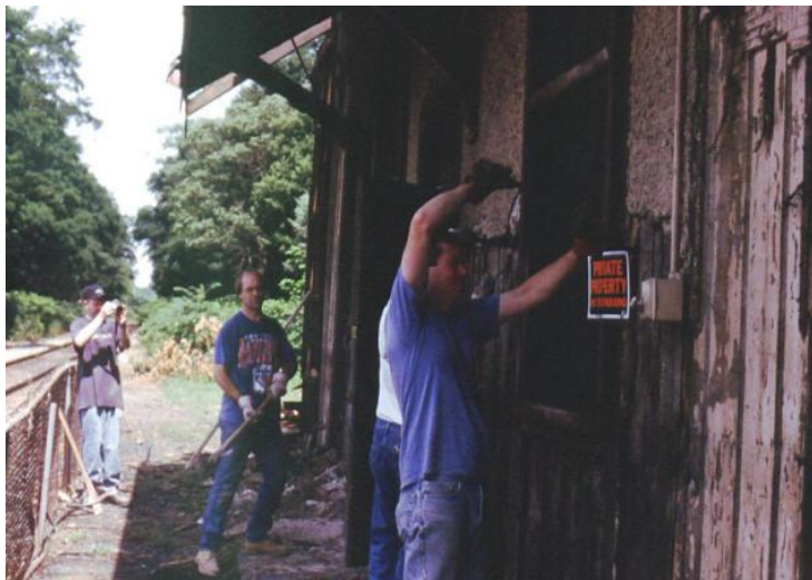
Remember the Saturday Morning Work Sessions? MSHC members Tim Moses, Rob Pisani, Glenn Fedkenheuer and Keith Smollin are shown removing stucco from the wall on the south side of the station on July 20, 2002. (Photo by Ed Kaminski)
